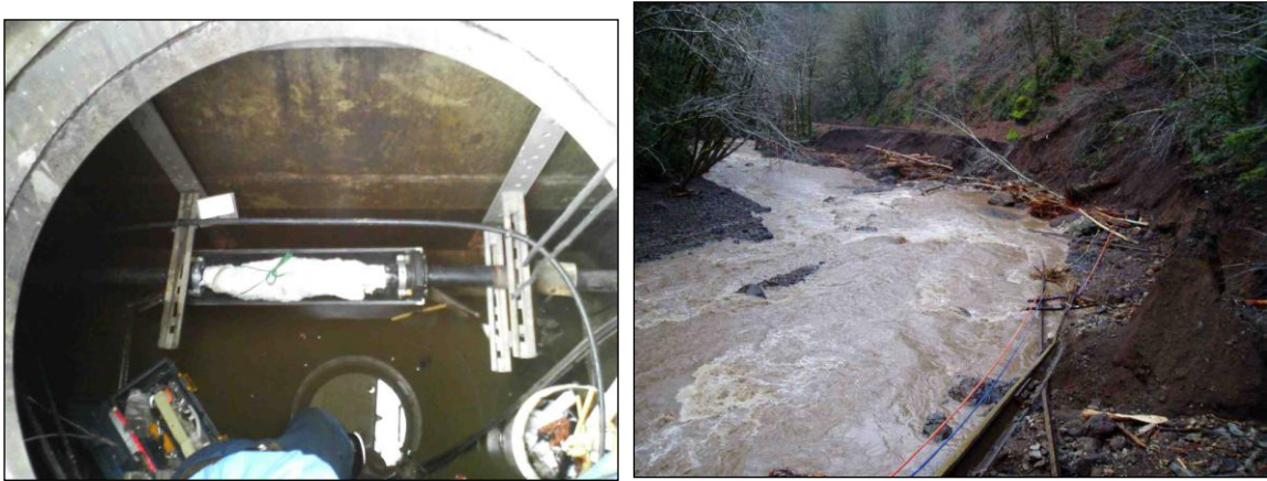
Figure 40. Damage to fiber optic cables: flooding degraded transmission when water leaked into a splice (left); ground failure damaged a cable laid along a railbed that washed out (right).
